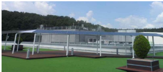
Solar power installation at Yongin Site
