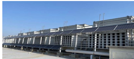
Solar power facility at Jukjeon Data Center
