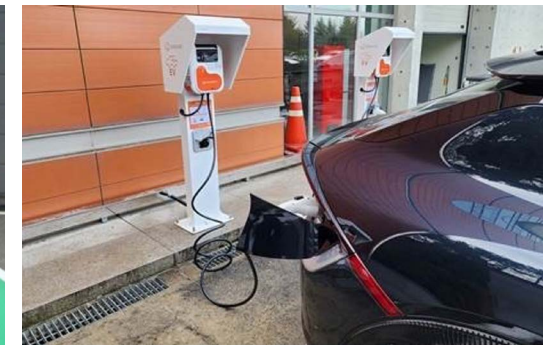
Electric vehicle chargers at Jukjeon Data Center
