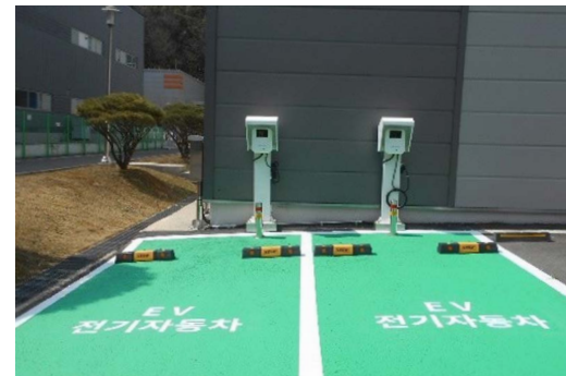
Electric vehicle chargers at Yongin Site
