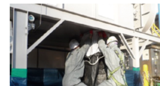
Replacing activated carbon in adsorption towers (first and second half of the year)
